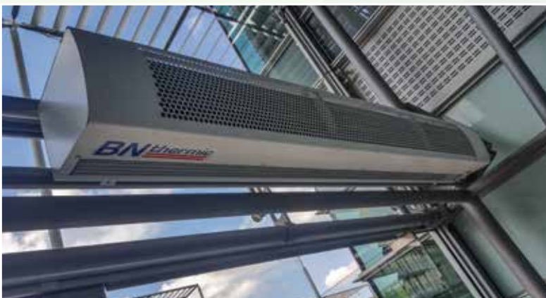
An air curtain looking the part in a prestige London office building
